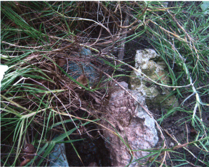
Ends of 2-8" emergency discharge pipes
