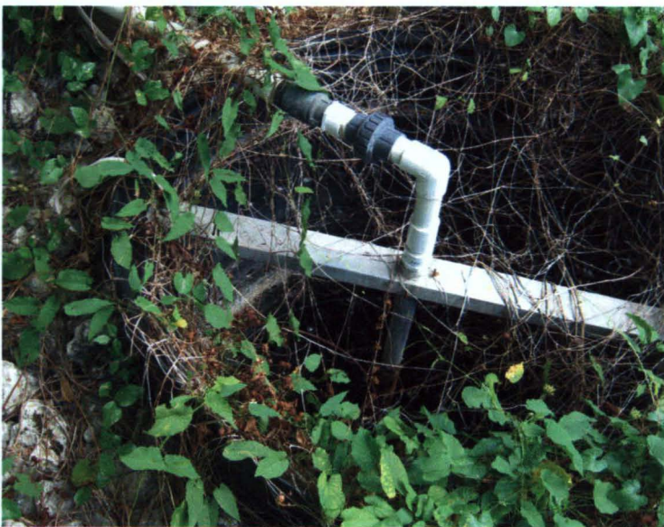
Pump in Springs at Freshwater Pond
