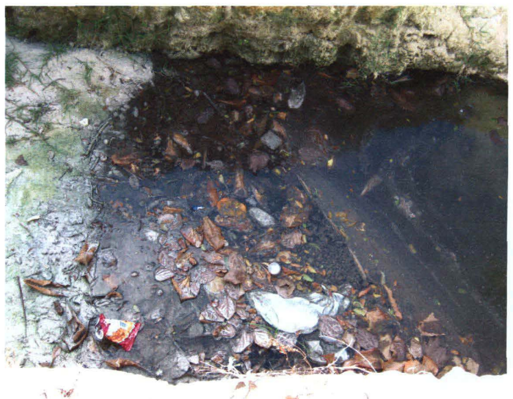
Debris in canal at Sluice Gate
